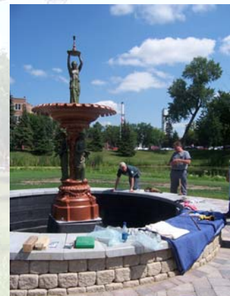
Electricians, Jerry Braaten & John Deitz "What happens when water & electricity mix?"
